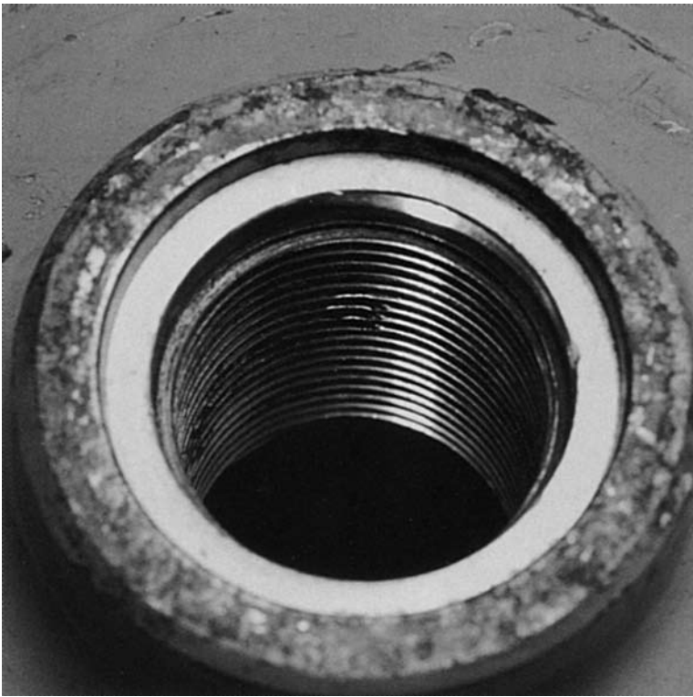
PHOTO 5. Damaged threads. This damage is easily seen with the naked eye, but the thread area is dirty and first needs cleaning (see NOTE 9), before proceeding with the visual inspection of the thread area.
