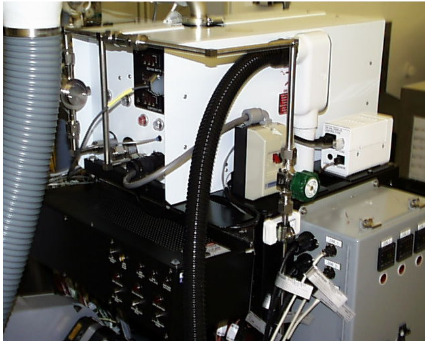
HGS System mounted on top of the AC Tower
