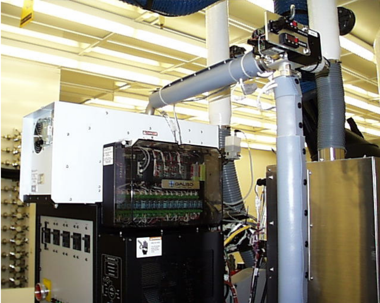
Process Manifolding to HGS-101 Unit
